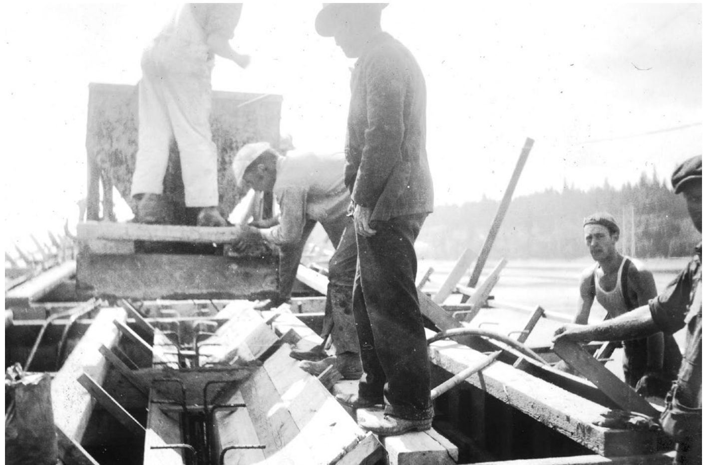
Workers pouring concrete during construction of the bridge. Washington State Archives, WSDOT Records
